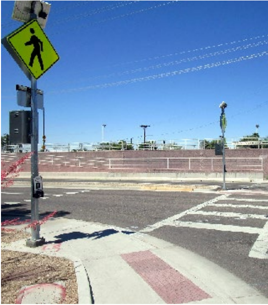
Rectangular Rapid Flashing Beacon
