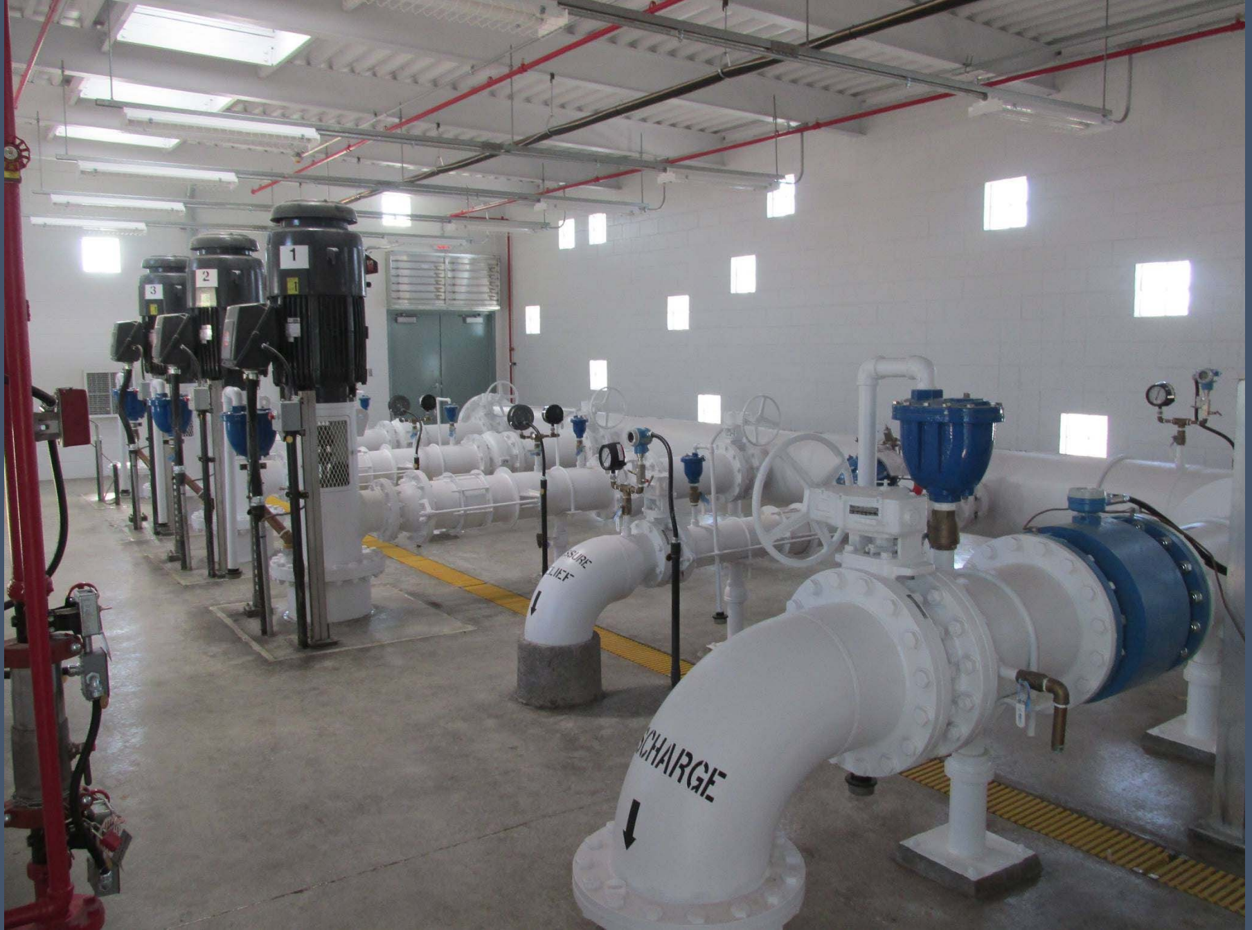
Site 71 Well Site & Booster Pump Station
