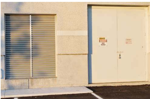
Exterior access transformer vault door and ventilation
