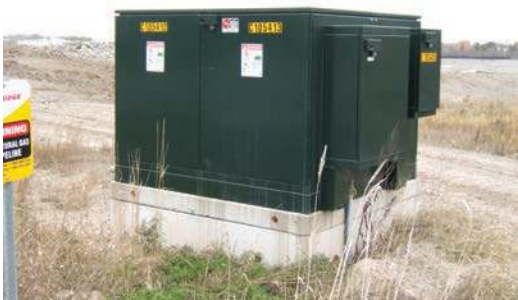
Pad mounted switchgear
