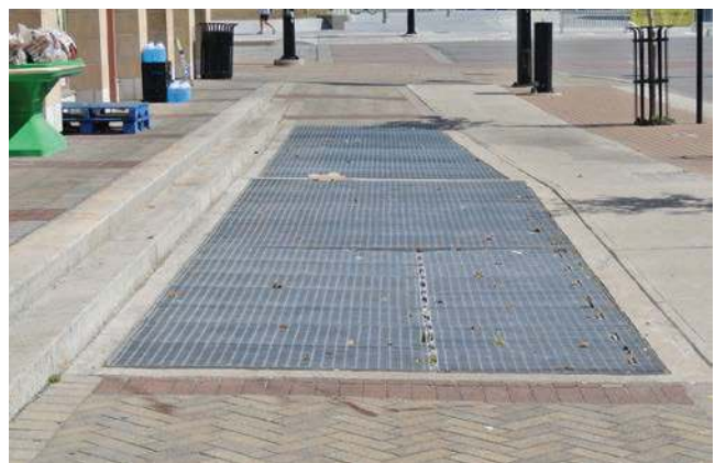
Sidewalk grates used for transformer access and ventilation
