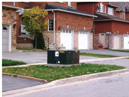
Pad mounted transformer
