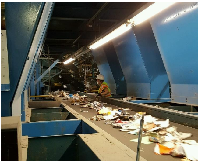
Processing line at the Salt River Pima-Maricopa Indian Community's Material Recycling Center
