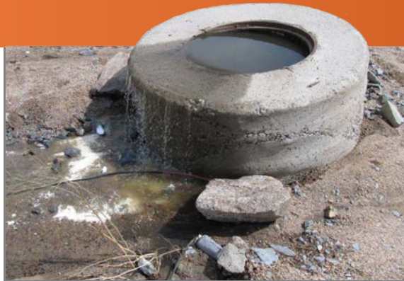
Sanitary sewer overflow caused by FOG
