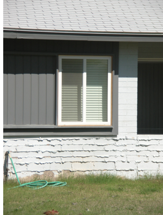
The boxed window appearance and wall materials have been retained but the pattern of glass panes has been changed when the window was replaced.
