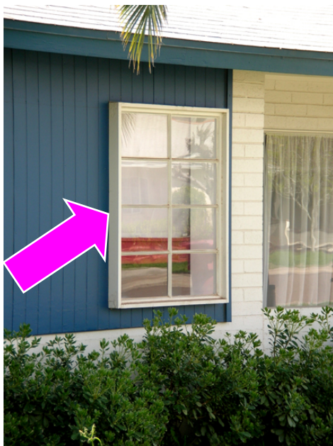
Allied used vertical and horizontal strips of wood around the windows to create 'boxed windows'
