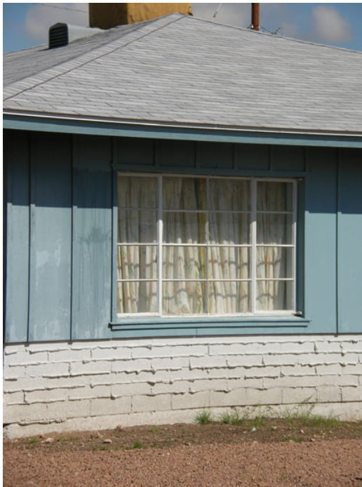
The original steel casement windows used in Ranch style homes have a variety of types and pattern. The above windows has sixteen rectangular shaped panes and the side windows can be cranked open.
