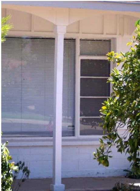
Replacing wooden posts with decorative columns with arches between the columns changes the historic porch details.
