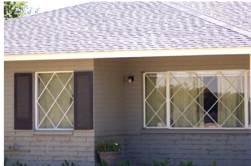
Some steel casement windows in Village Grove have the decorative diamond pane pattern. Shutters also flank some windows on the front façade.
