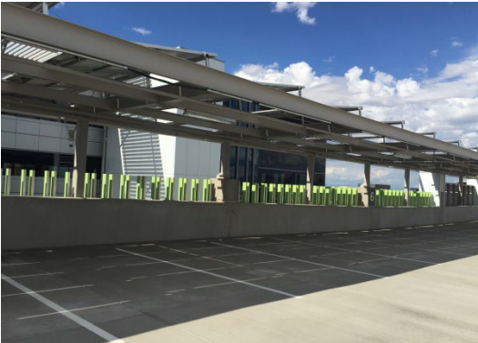
Solar PV parking shade canopy at top level of garage.
