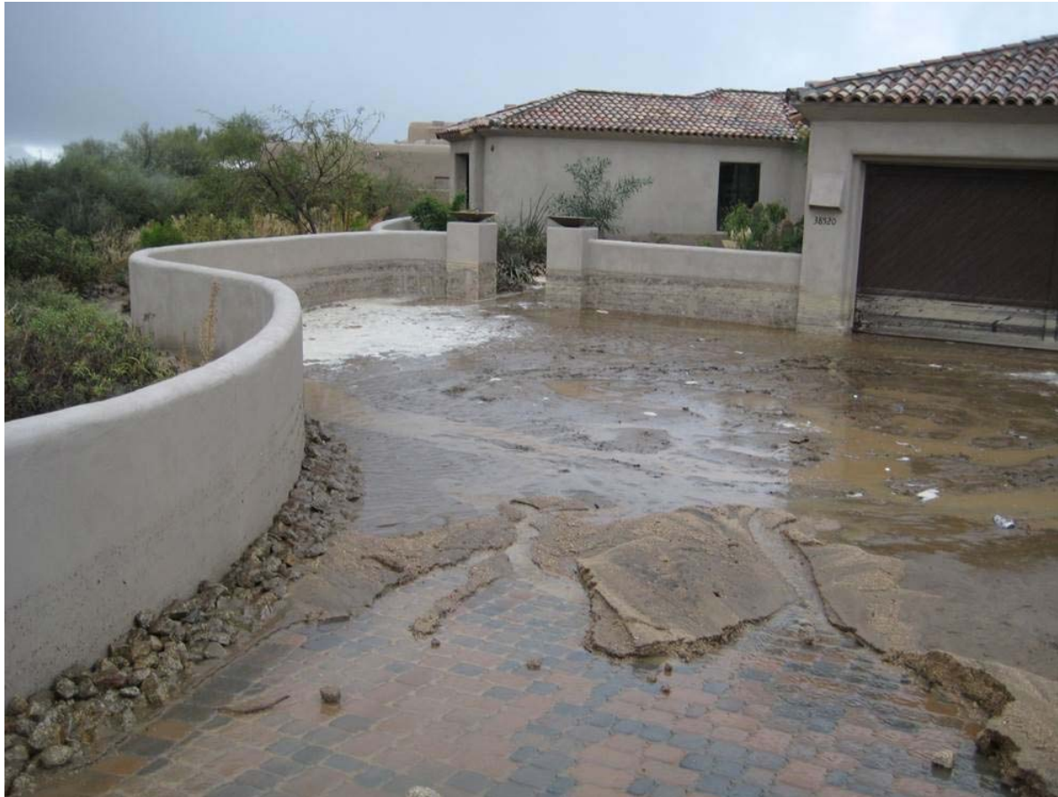
Desert Mountain subdivision $250k storm damage – Aug. 2014 storm
