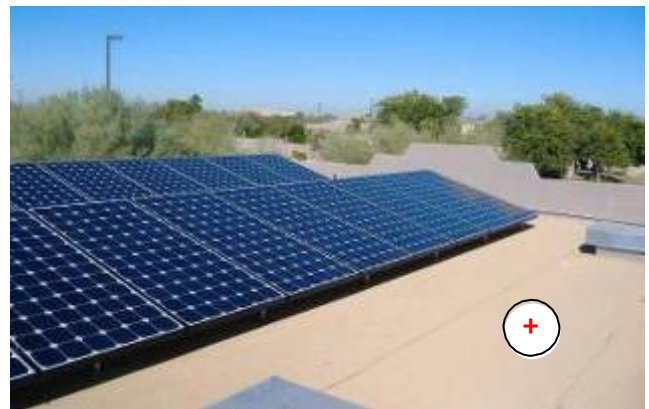
Solar panels on flat roof with parapets.
