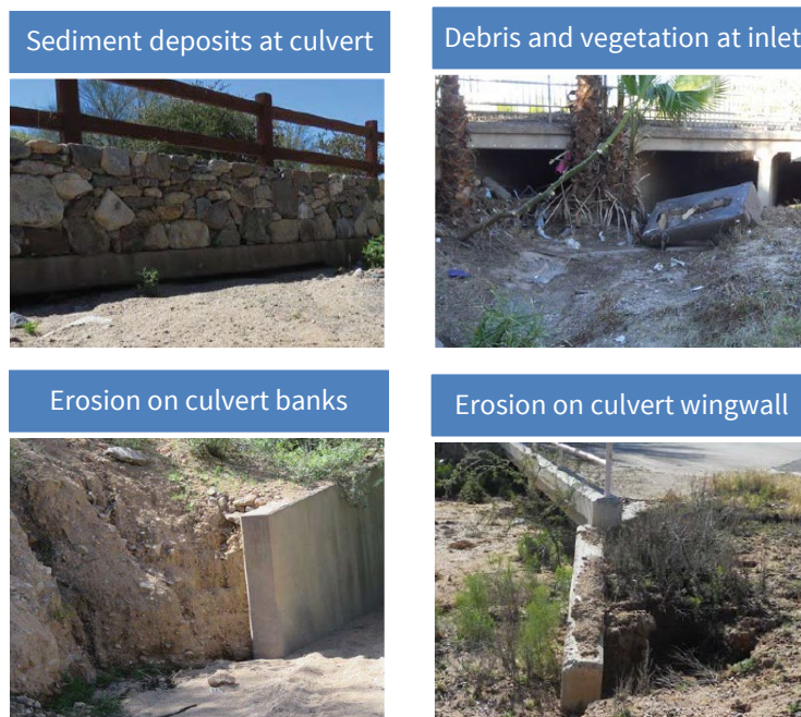
Figure 9. Maintenance Needs Not Identified in City Drainage Asset Inspections
