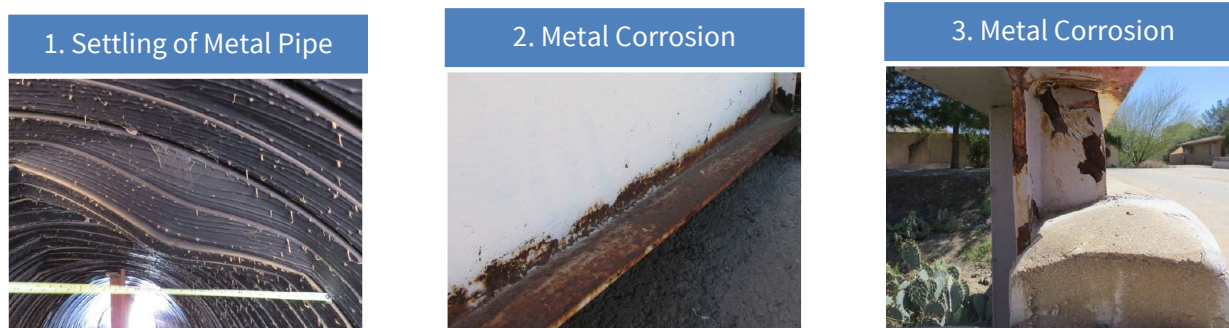
Figure 8. ADOT Bridge Inspections with “Structurally Deficient” Classifications
