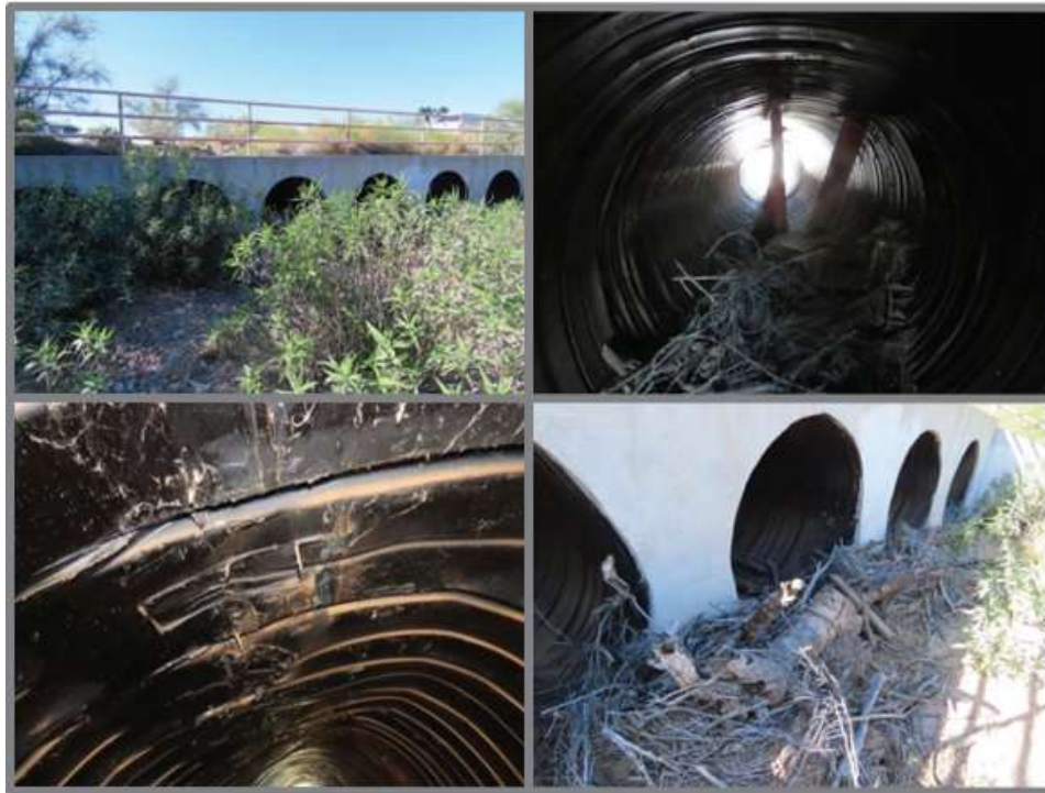
Figure 6. Culvert rated in poor condition on 117 th Way needs repairs and maintenance.
