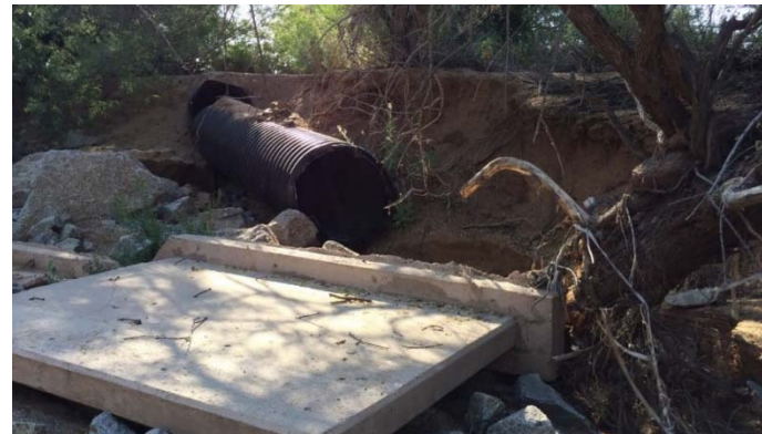
Stormwater Damage Desert Mountain Golf Course Clubhouse Photo taken June 2015
