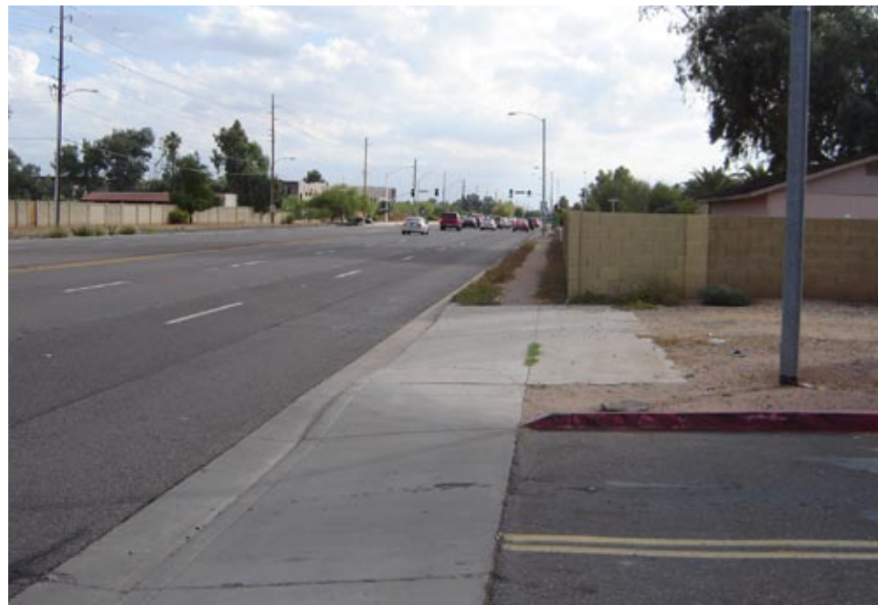
Abrupt sidewalk ending near Sutton Drive disrupts continuous pedestrian circulation
