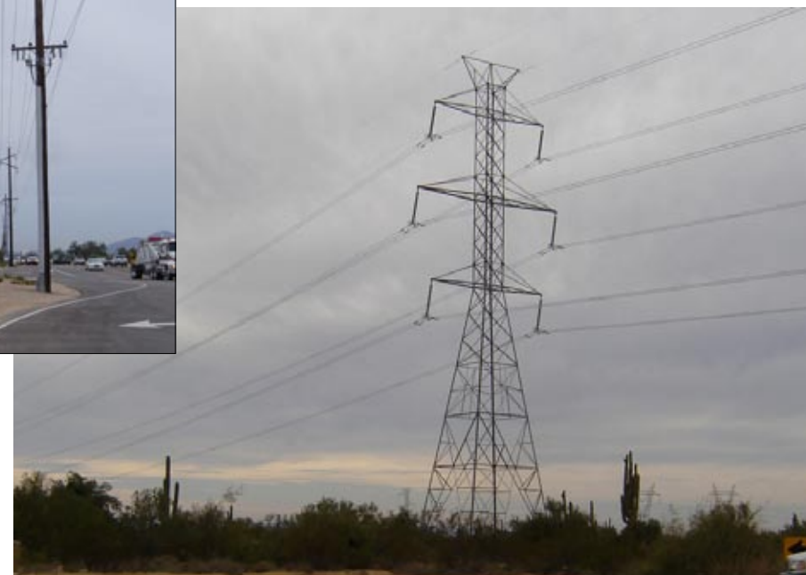
High voltage transmission towers and lines cross the corridor in multiple locations
