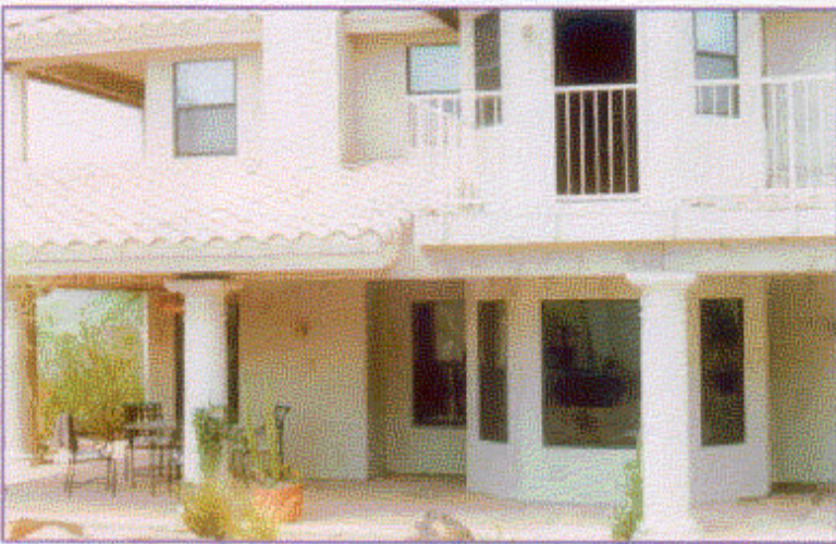
The rear of the large structure. Note little evidence of any fire. (CS7-2)
