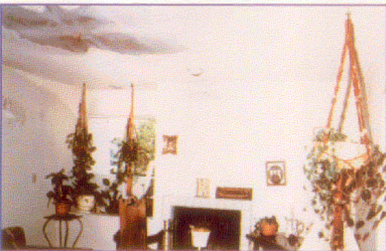
An overall view of the main living area. Only minor water damage to ceiling, walls, and interior furnishings. Note the wall wetting action from the specially designed residential sprinkler head. (CS2-3)
