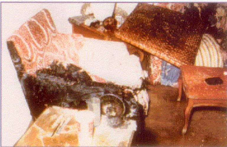
Point of origin is on the left side of the chair. Note minimal damage to surrounding combustibles. (CS2-2)
