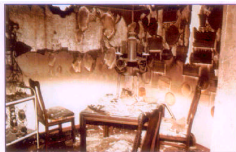
Although the fire never reached the dining area, smoke and heat damage were significant. (CS5-4)
