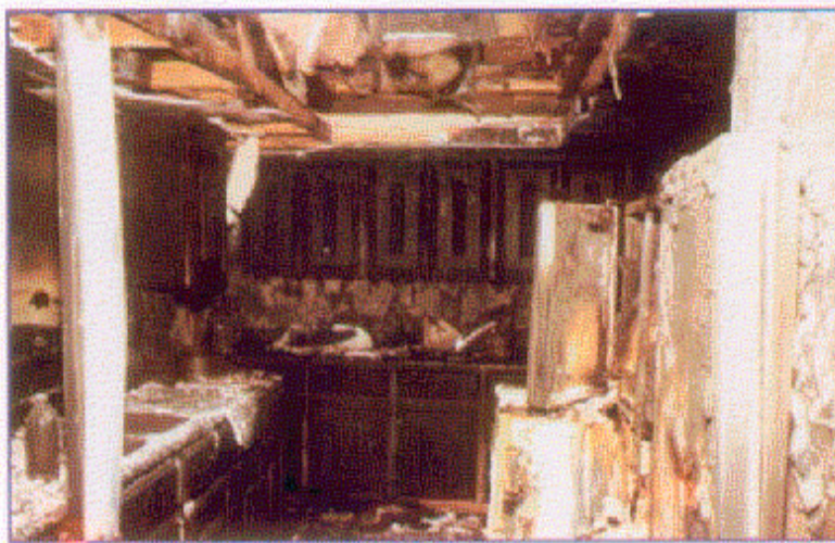
Extensive damage to the kitchen area. This is where suppression crews halted the extension of the fire. (CS5-3)
