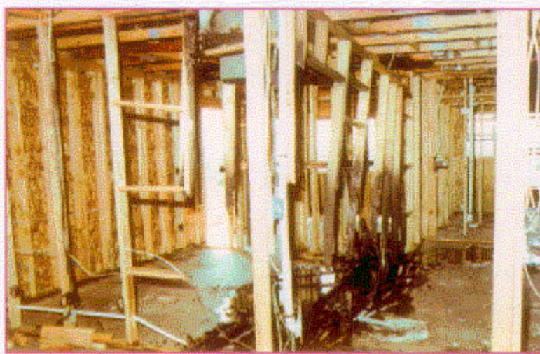
The area of the flammable liquid pour. Note the placement at the base of the highly combustible framing. (CS8-2)
