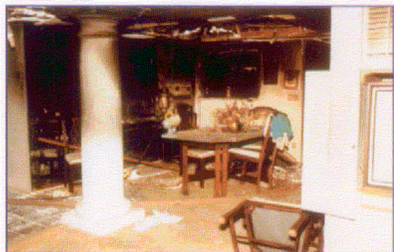
Smoke and heat damage extended throughout the living area despite the fact that the fire never extended into the area. (CS5-5)
