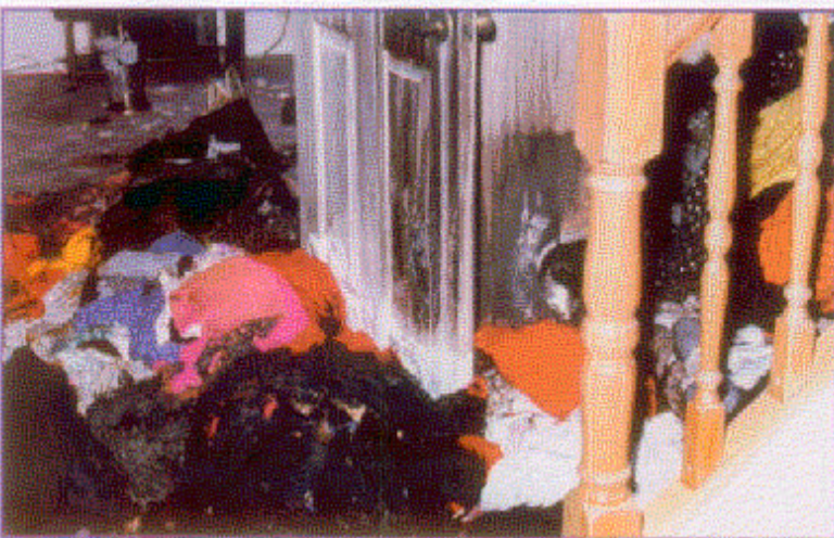
The interior hall and stair case. The clothes and other combustibles were combined with flammable liquid to accelerate the fire. There was heavy soot and smoke damage but very little structural damage as a result of the fire. (CS6-3)
