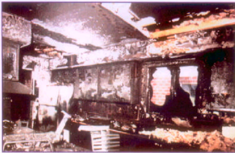
An example of heavy fire extension into the kitchen area. (CS9-4)
