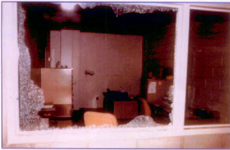
A closeup view of the shattered window and interior damage from projectiles launched during the explosion. (CS1-7)
