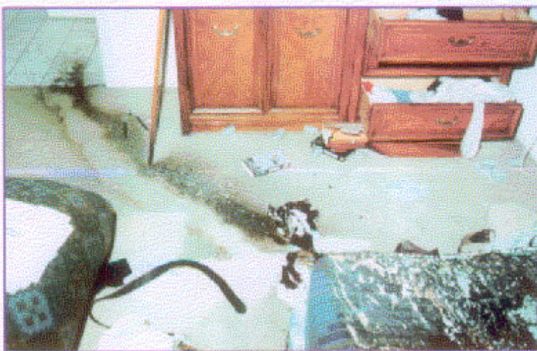
Another view of the poured gasoline as it extends out of the bedroom. Notice only minor damage from the flash fire prior to the sprinkler suppressing the flames. (CS6-4)
