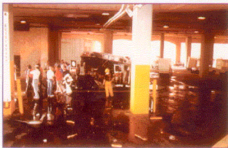
A closer view of the damage associated with the explosion. The sprinkler pipe remained intact. (CS1-6)
