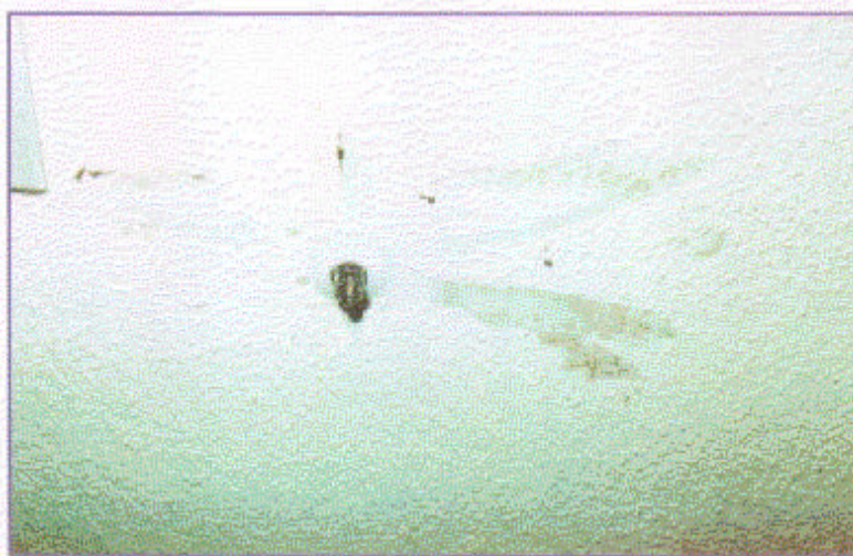
The activated sprinkler head caused only minor damage to the finish of the ceiling area. (CS6-2)
