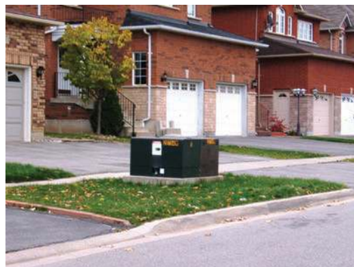
Pad mounted transformer
