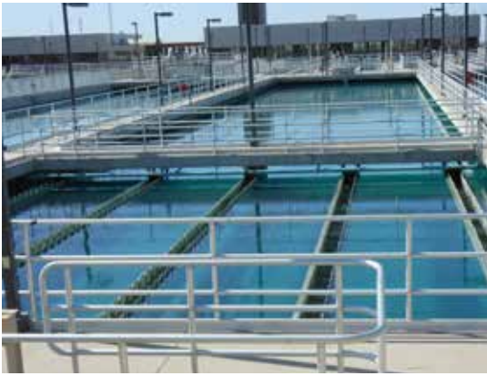
Water quality testing pools at Scottsdale Water Campus
