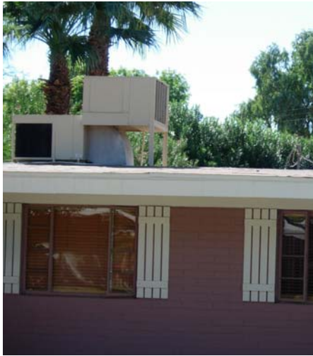
Roof mounted mechanical units have a major impact on the appearance of the house.
