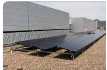
Alternative energy generation, such as solar power, can help reduce peak electricity demand and save on energy costs. Photo source: Henkel.
