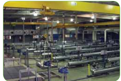
Chaparral Water Treatment Plant incorporates award-winning membrane filtration process.
