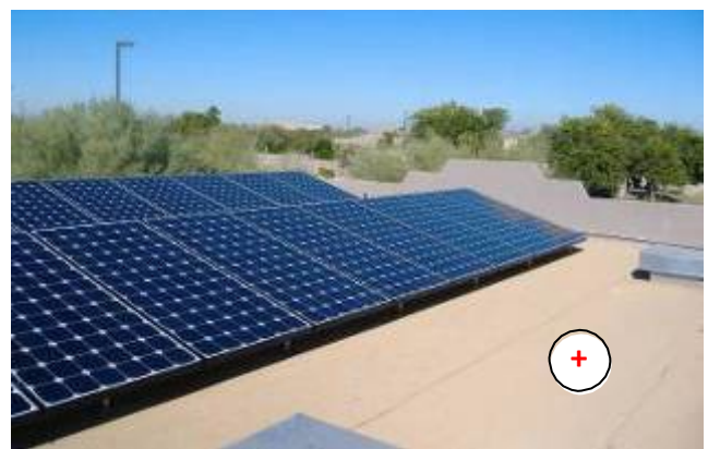
Solar panels on flat roof with parapets.
