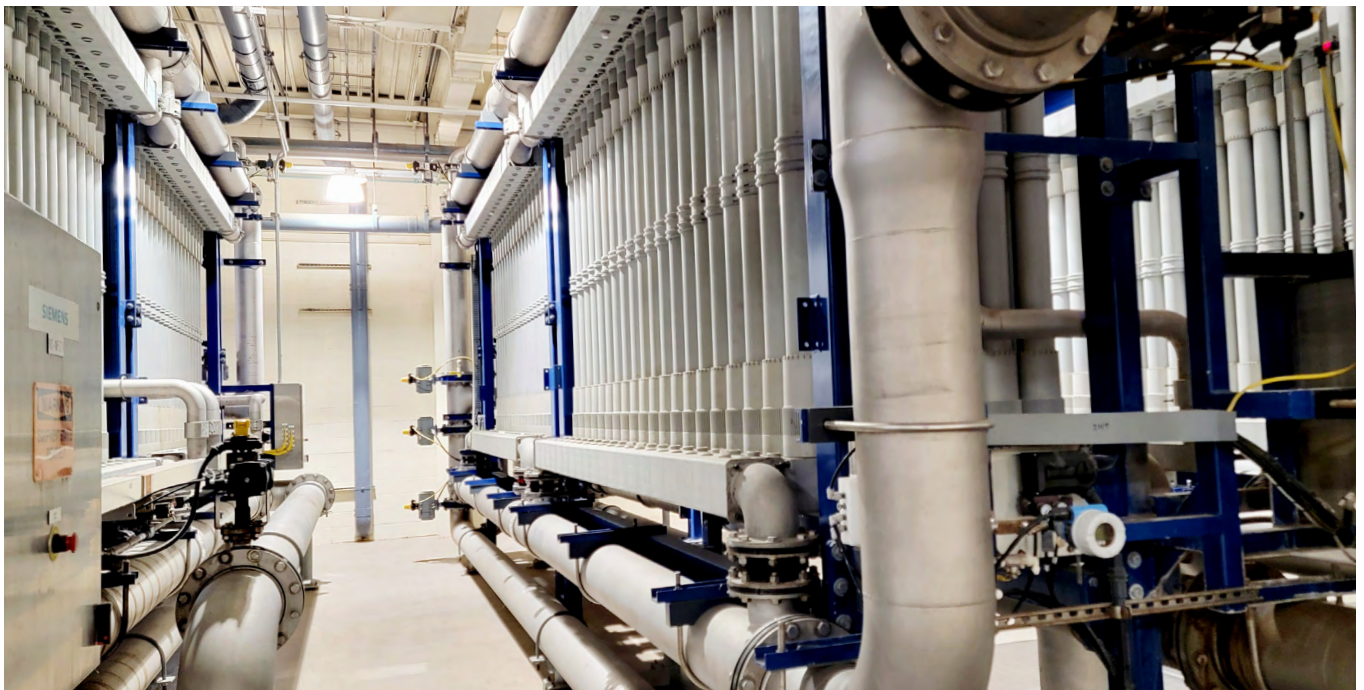
Ultrafiltration Facility at Advanced Water Treatment Plant: Membrane filtration process filters out viruses and bacteria, and pre-treats prior to Reverse Osmosis.
